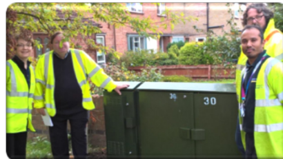
Pilot installation: Street cabinet with G.fast sidepod 2
